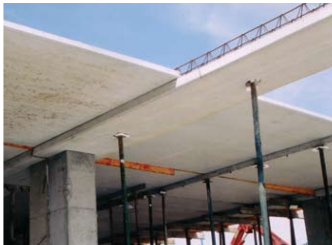
Fig. 4: Dropped precast slabs spanning between the columns partially support the precast slabs spanning in the other direction
