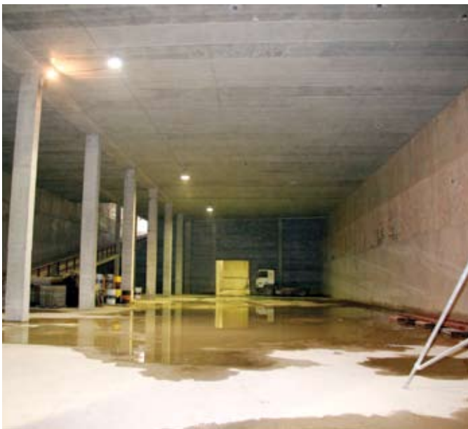
Fig. 7: Interior view of the 17 x 55 m (56 x 180 ft) column-free area shown in the structural floor plan in Fig. 6
