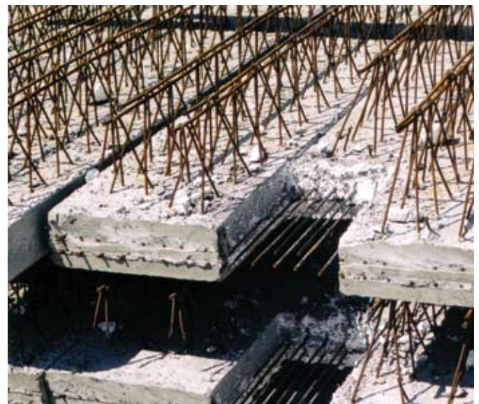
Fig. 5: The slab blockout shown here is used in a dropped slab panel spanning between columns and allows the column vertical reinforcement to pass through the precast panel
