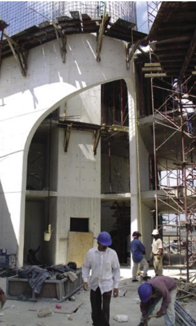
View of cutouts in the central core structures at the main lobby level
