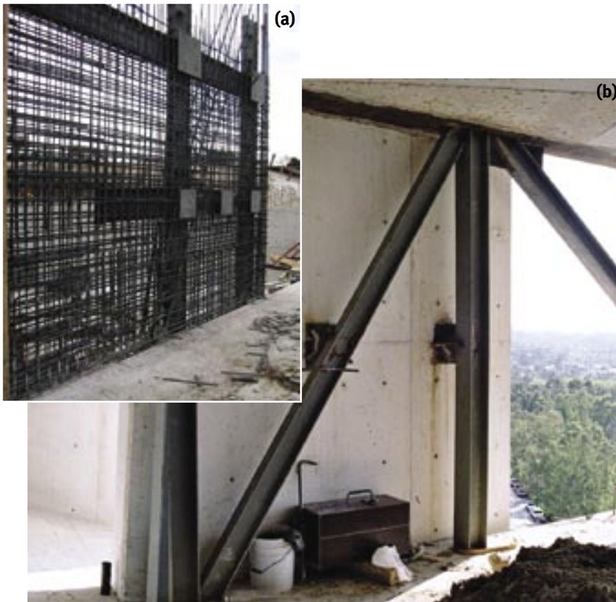
Fig. 6: Connection between the concrete walls of the central core and the steel trusses supporting the floor plates: (a) during construction; and (b) after installation of the trusses and floor
