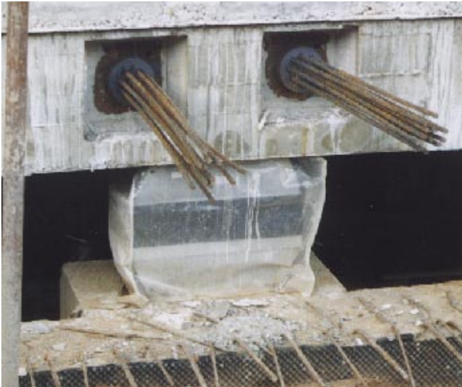
Fig. 6: Base isolation unit and post-tensioning anchorages
