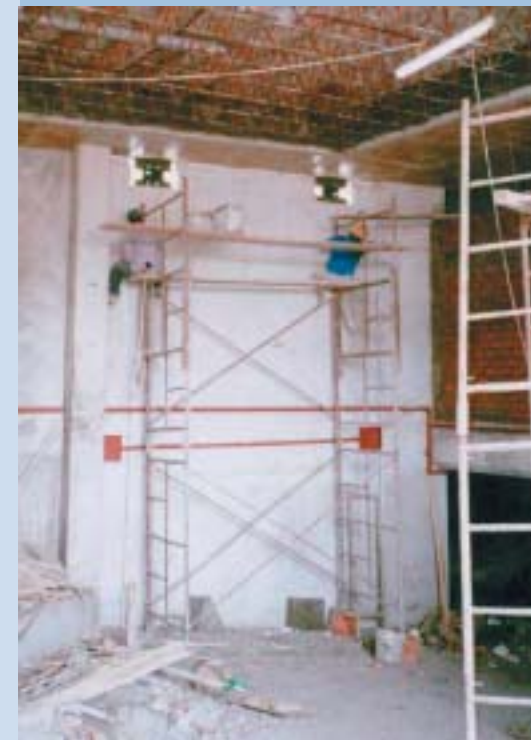
Casino building in Lima, Peru with BOZZO-GERB Dissipators
